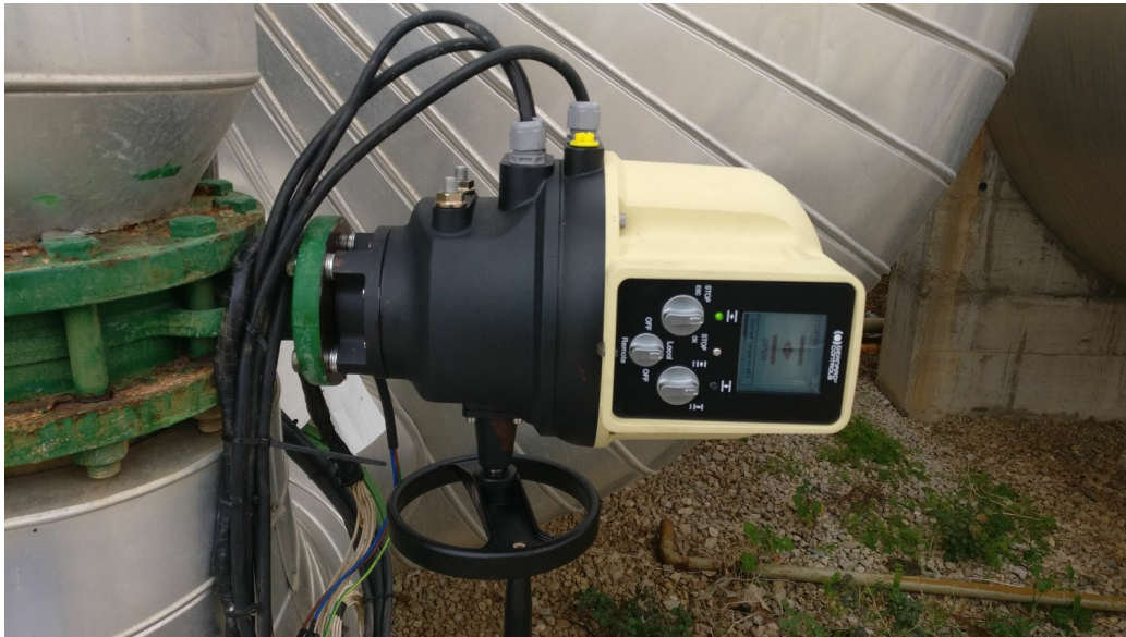
Figure 4.22: Valve actuator to control supply temperature
