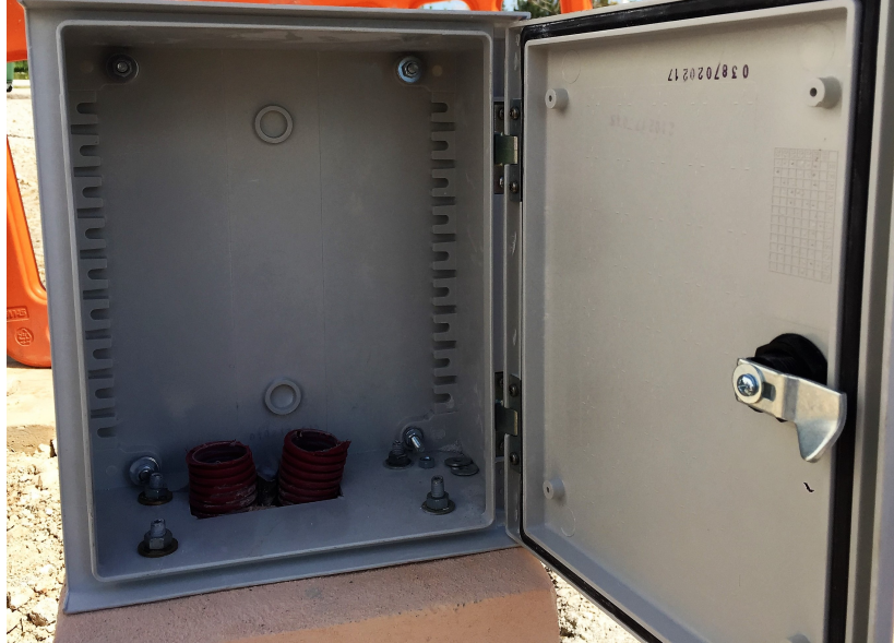
Figure 5.1: The power supply wires (left red tube) and the pressure tubes (left red tube) inside the IP57 box (E2).
